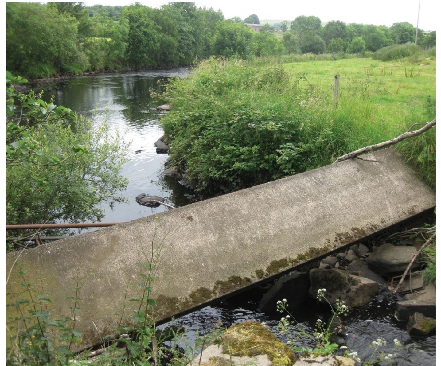
Fig. 5 – Example of an Existing Item where 'Needs replaced' is recorded
